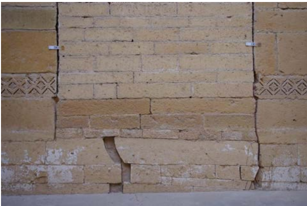
Figure 7. large cracks between the masonry infill and the original structure, 2018
