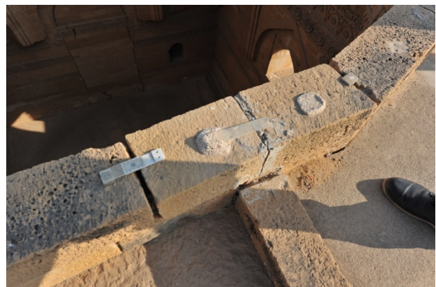
Figure 2. Old plaster and glass crack monitors were discovered on several monuments, but there were no written records
