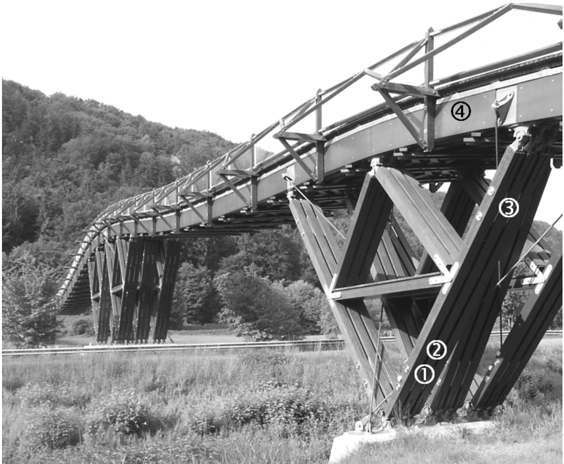
Figure 7.3-3. Self-supporting pedestrian timber bridge in Essing, made from Norway spruce gluelam: ① Bottom nail plates, ② region above bottom nail plates for installation of measuring points remote from the nail plates, ③ upper nail plates, ④ main trusses covered with plywood.
