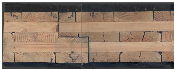
Fig. 15. Checking, cupping, and general deterioration of the panel observed in edge B near the half-lap joint after weathering.
