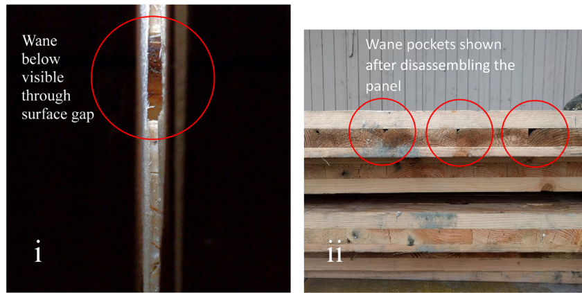
Fig. 12. Wane in the CLT panel. (i) — Wane clearly visibly through surface gap. Note cracks in resin. (ii) — Wane visible in the second ply after disassembly of the half-lap joint.
