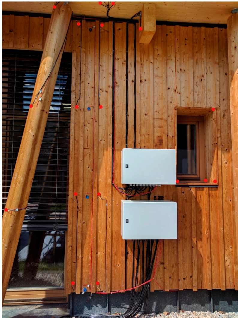
Figure 2. Position of wood moisture and temperature sensors on the façade of the Annex. The red dots indicate locations of the measurements.
